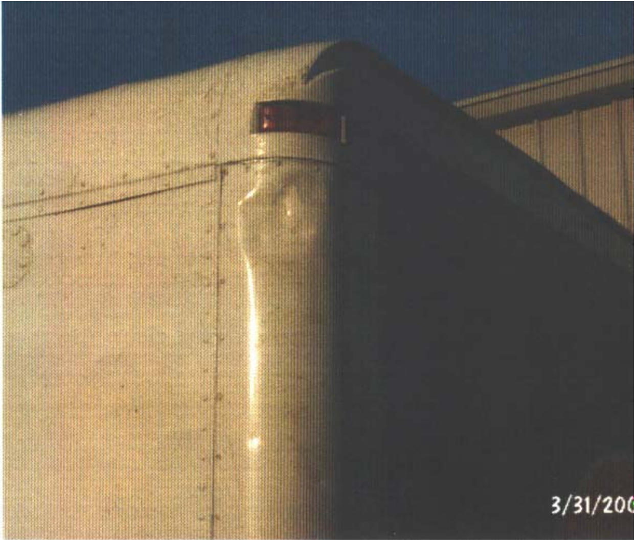
Picture of the dent caused by the cargo truck hitting the bucket with the traffic technician in it. (Photograph courtesy of employer)
