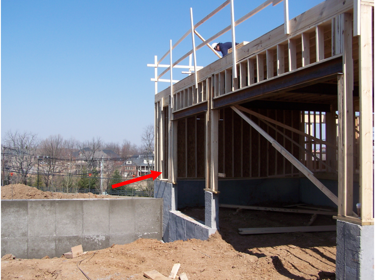
Corner of house where carpenters were to erect the wall. The concrete wall was not there at time of incident.
