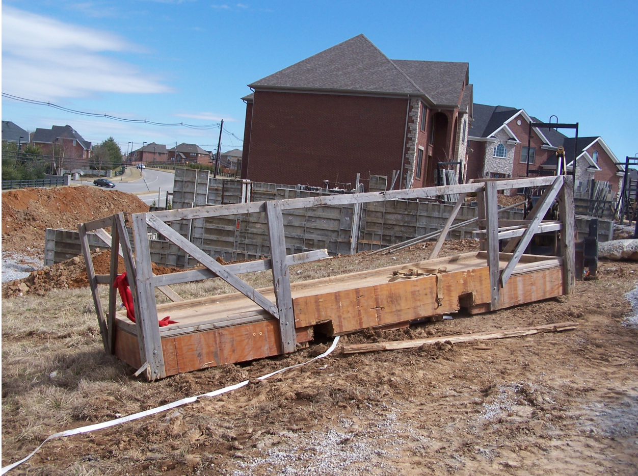
Picture of homemade platform involved in this incident. Notice railing and cleats.
