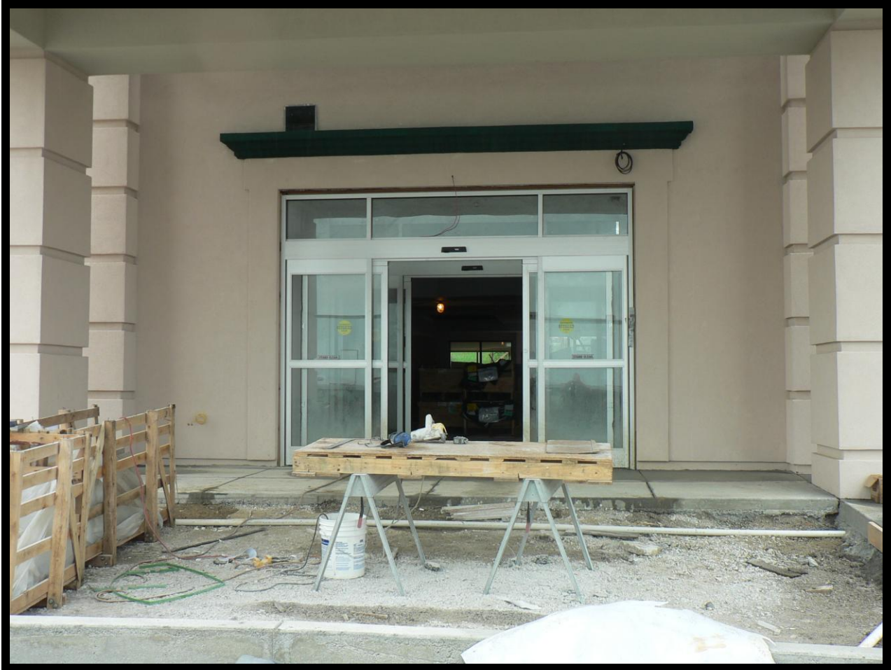
Photograph of onsite trim area outside main entrance. Photograph courtesy of local police.
