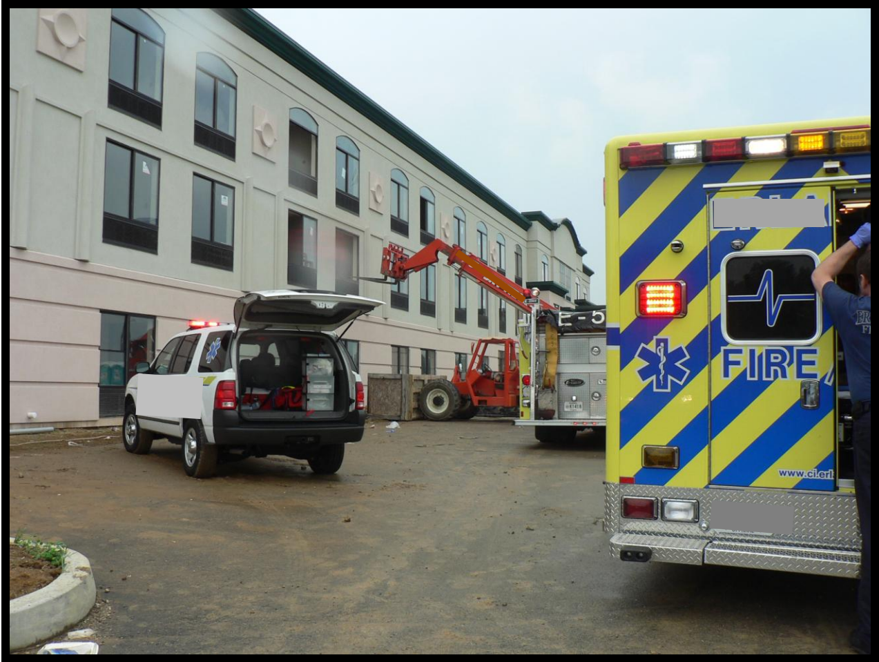
Photograph of forklift raised to 2 nd story window as it was during the incident. Photograph courtesy of local police.
