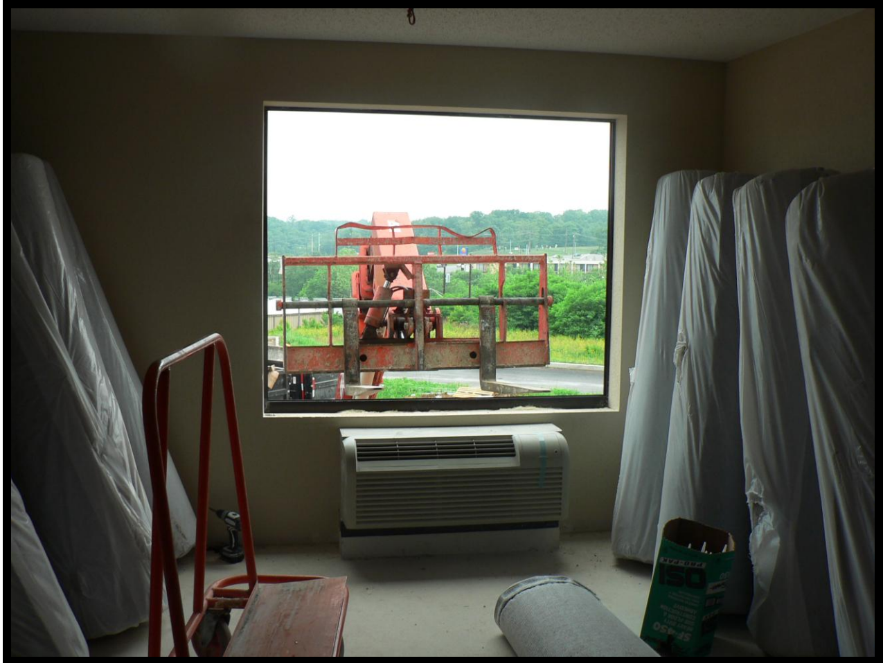
Photograph of window accessed to unload granite from construction box, forklift used to lift construction box with granite, and a granite cart. Photograph courtesy of local police.
