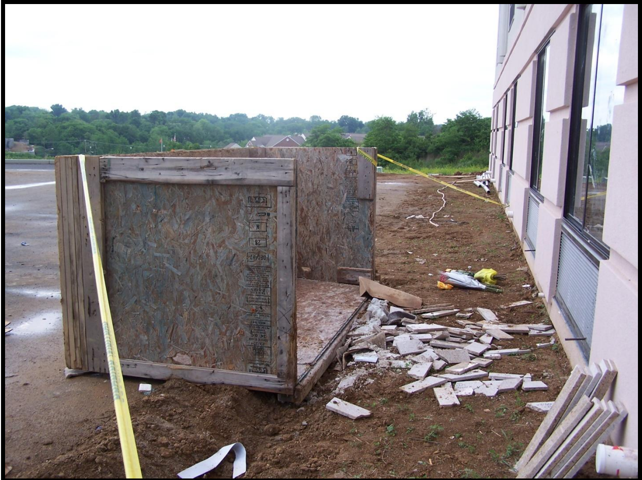
Photograph of construction box involved in this incident. Photograph property of KY FACE program.
