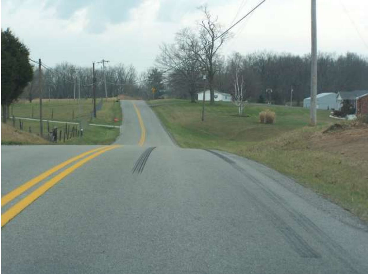
Photograph of location where car topped hill and lost control. Picture property of KY FACE.
