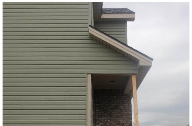
Photo 2: Side angle of the porch area (photo courtesy of KY OSHA).
