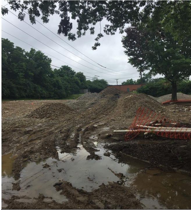
Photo 1: Incident site. Photo property of KY FACE.
