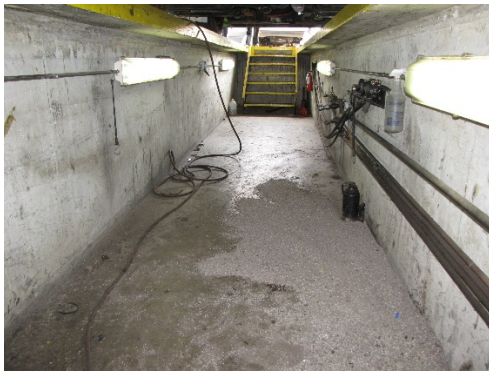
Figure 4. View of the pit in which the victim was working at the time of the incident.
