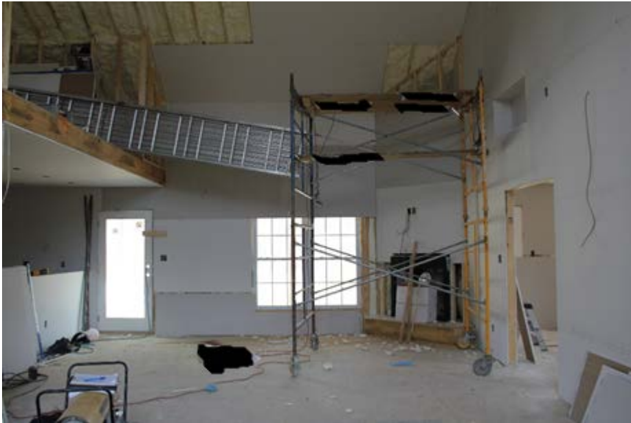
Figure 1. Scaffold and plank from which the victim fell
