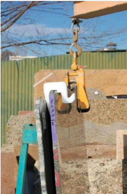
Photo 6: Positioning Relative to Rack [Wehausea.com]
