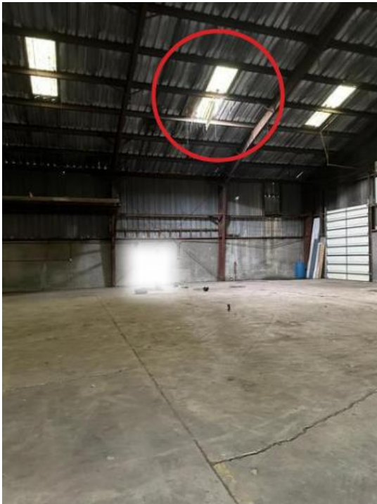
Photo 4. Red circle identifying the polycarbonate skylight the victim fell through.
