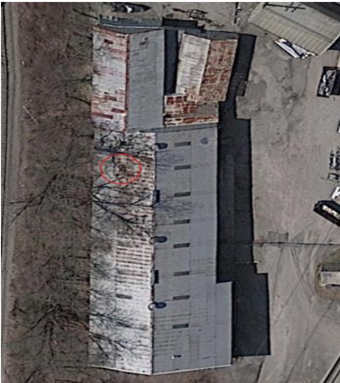
Photo 1. Google Earth image of building where the incident occurred. The red circle indicates the skylight involved in the incident.
