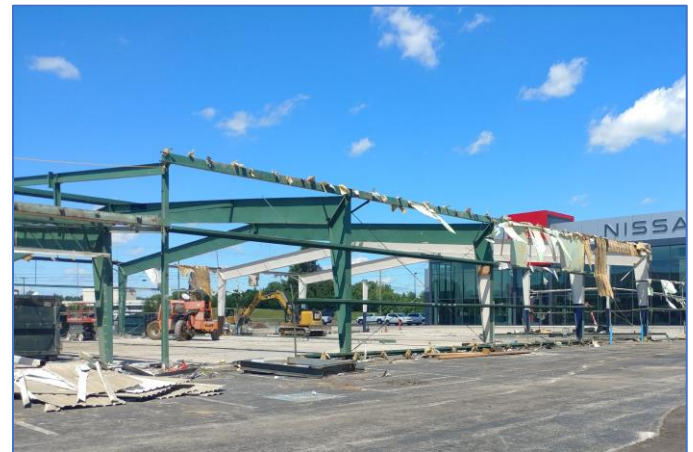
Photo 4. Building framework remaining at time of FACE site visit (Property of FACE program)
