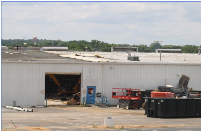
Photo 3. Building undergoing demolition on day of fatal incident (Courtesy of KyOSHA)
