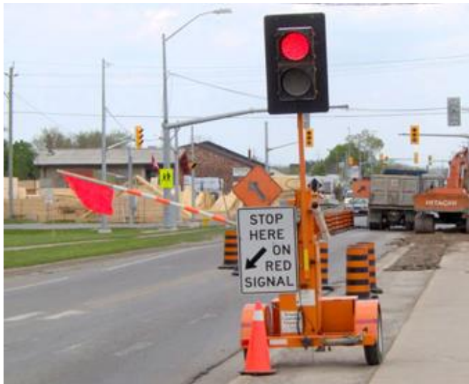
Photo 15. Photo of AFAD. Photo retrieved from and property of temporarytrafficsignals.com .
