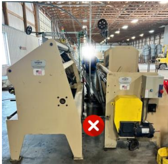
Photo 6. Red X indicates prohibited area where the employee entered and the fatal event occurred. Photo property of Kentucky FACE.
