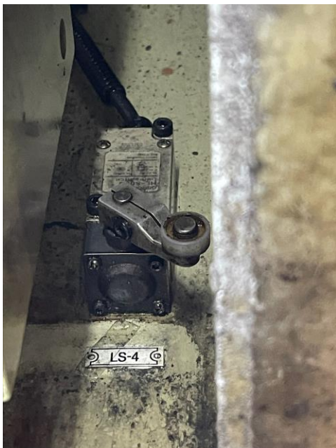
Image 4. Access Door Interlock (Property KY FACE)
