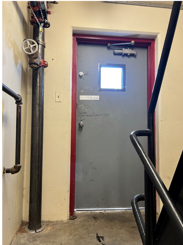
Photo 4. Roof access door at the location where the event occurred. Photo property of KY FACE.
