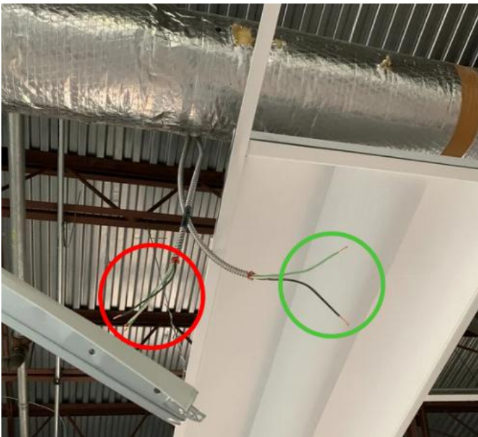
Photo 3: Unenergized wire (green circle) installed by the victim and energized wire contacted by the victim (red circle), which resulted in the fatal injuries. Photo obtained via open records request.
