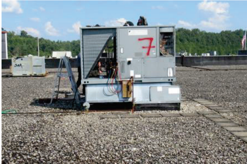
Photo 2. The Daikin commercial HVAC unit involved in the incident. Photo obtained via open records request.
