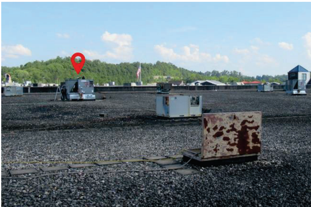
Photo 3: Roof where the incident occurred. Red location marker identifies the HVAC system involved. Photo obtained via open records request.
