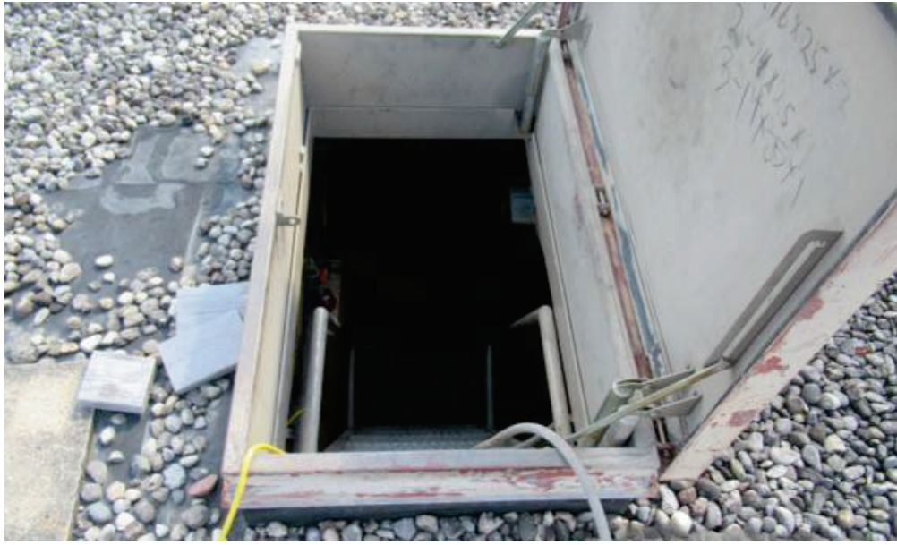
Photo 4: Roof access point utilized by the victim. Photo obtained via open records request.
